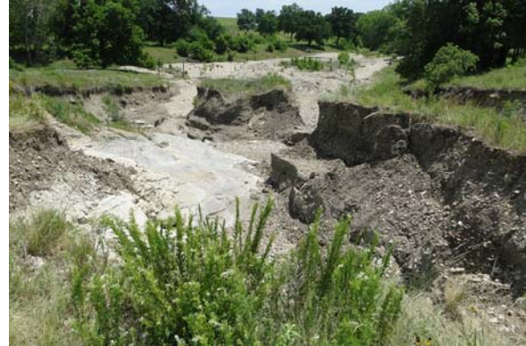
Damage from auxiliary spillway flow on watershed dams
